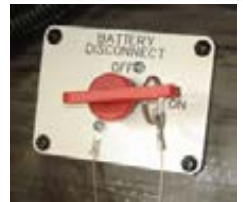
Battery Disconnect Switches may vary by model
